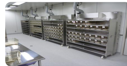
Animal research facility with full AAALAC accreditation with HVAC controls
